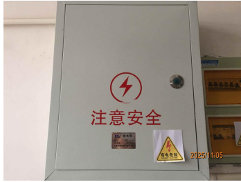
electrical control panel marked with warning sign.JPG
