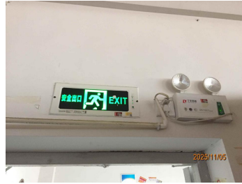
exit sign and emergency light.JPG
