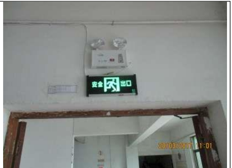
Emergency and exit sign light
