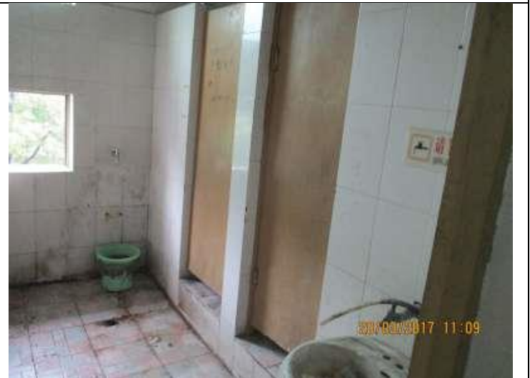
The toilets were not clean
