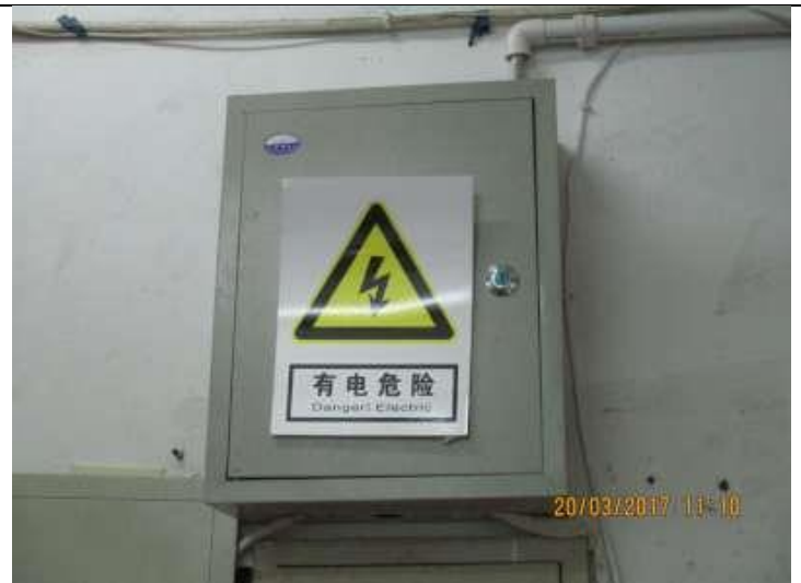
Safety electrical breaker
